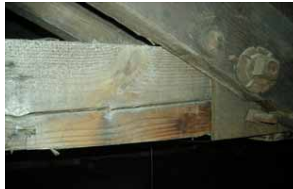
Figure 4 – Splitting in Bottom Chord
