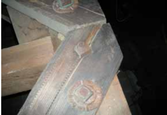
Figure 5 – Splitting in Diagonal @ Bolts
