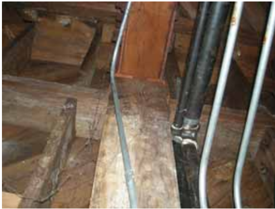
Figure 17 - Interior View of Double 2x Top Plate w/no Connection to Post
