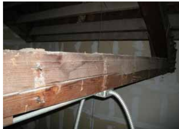
Figure 10 - Bottom Chord Splitting
