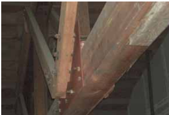
Figure 6 - Separation @ (n) Vertical and (e) Bottom Chord
