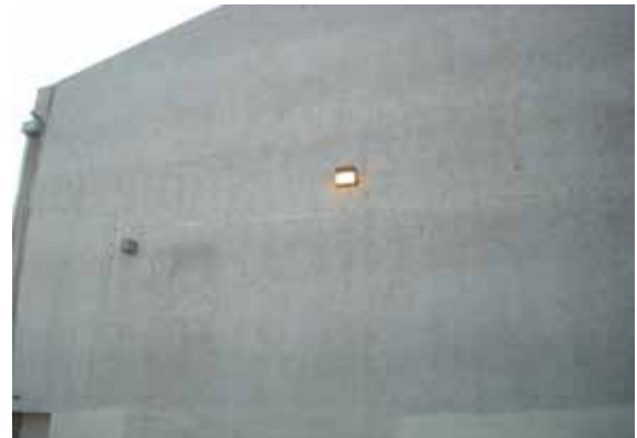
Figure 16 - East Exterior Elevation w/Horizontal Crack in Plaster
