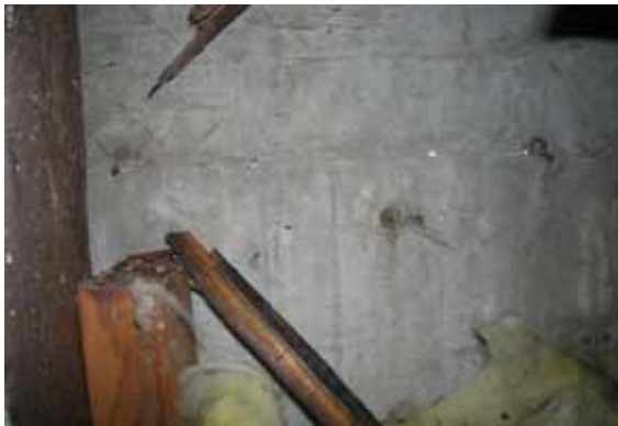
Figure 19 - Figure 18 - Interior View of Exterior 2x8 Wall w/Missing Sheathing and Delaminated Plaster
