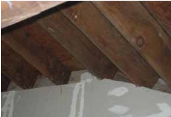
Figure 8 - Separation @ Roof Joists and Bearing Wall
