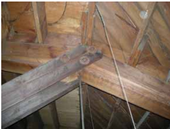
Figure 9 - Severe Splitting in Top Chord and Diagonal
