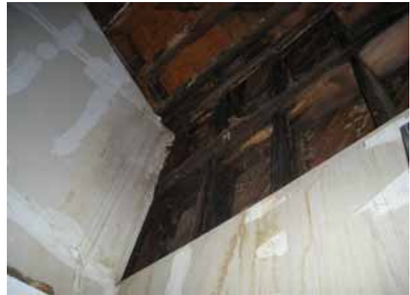
Figure 18- Interior View of Water Damaged Framing @ South/East Corner
