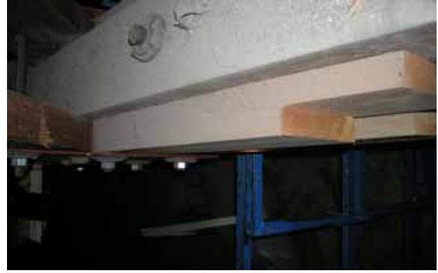
Figure 13 - Side View of (n) Repair at Bottom Chord
