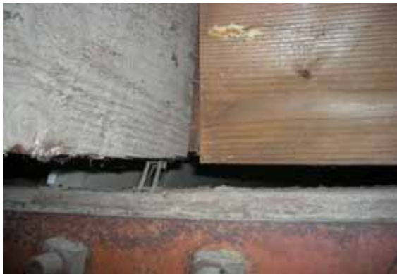
Figure 3 – Non-bearing Separation @ Top Chord & Roof Joist
