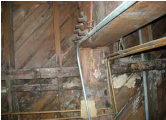
Figure 11 - Double Top Plate (hinge) at Truss and Water Damage
