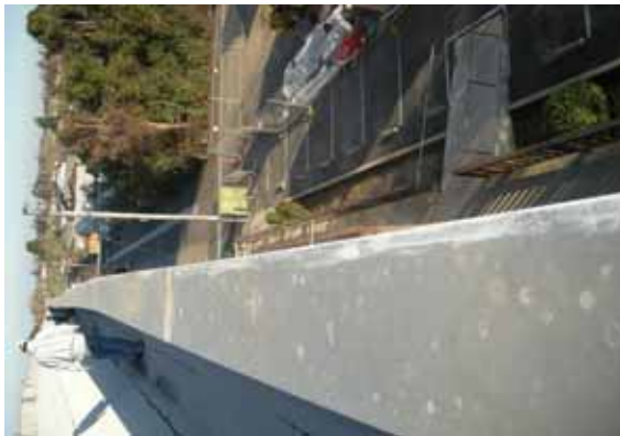
Figure 15 - Rooftop View of Bowing in South Wall
